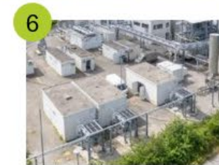
Grid injection plant
