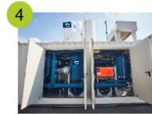
Liquefier and e-LNG filling station
