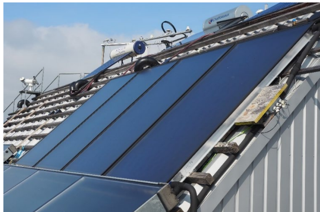
Figure 52: The four collectors of the demonstrator DBS mounted on the roof in parallel.
