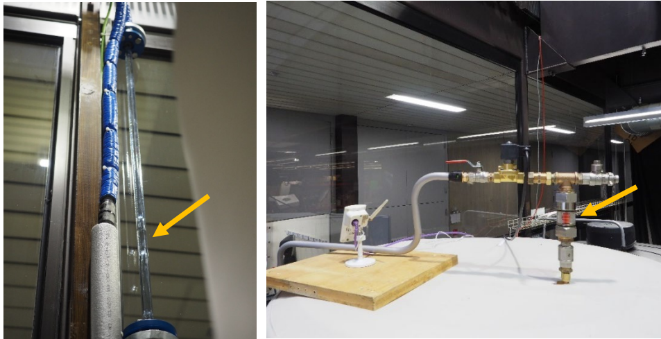
Figure 55: Transparent pipe section (see arrows) of the solar loop for visual observation of gases within the flow.
