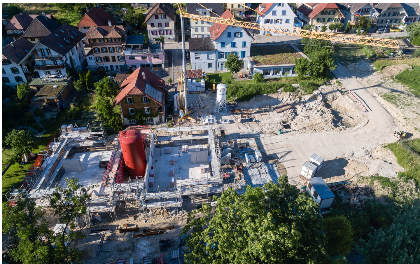
The apartment building in Huttwil contains a hot water storage tank (red tank) with a capacity of 110 m 3 ; it brings solar heat from summer into the winter months. Photo: Jenni Energietechnik AG
