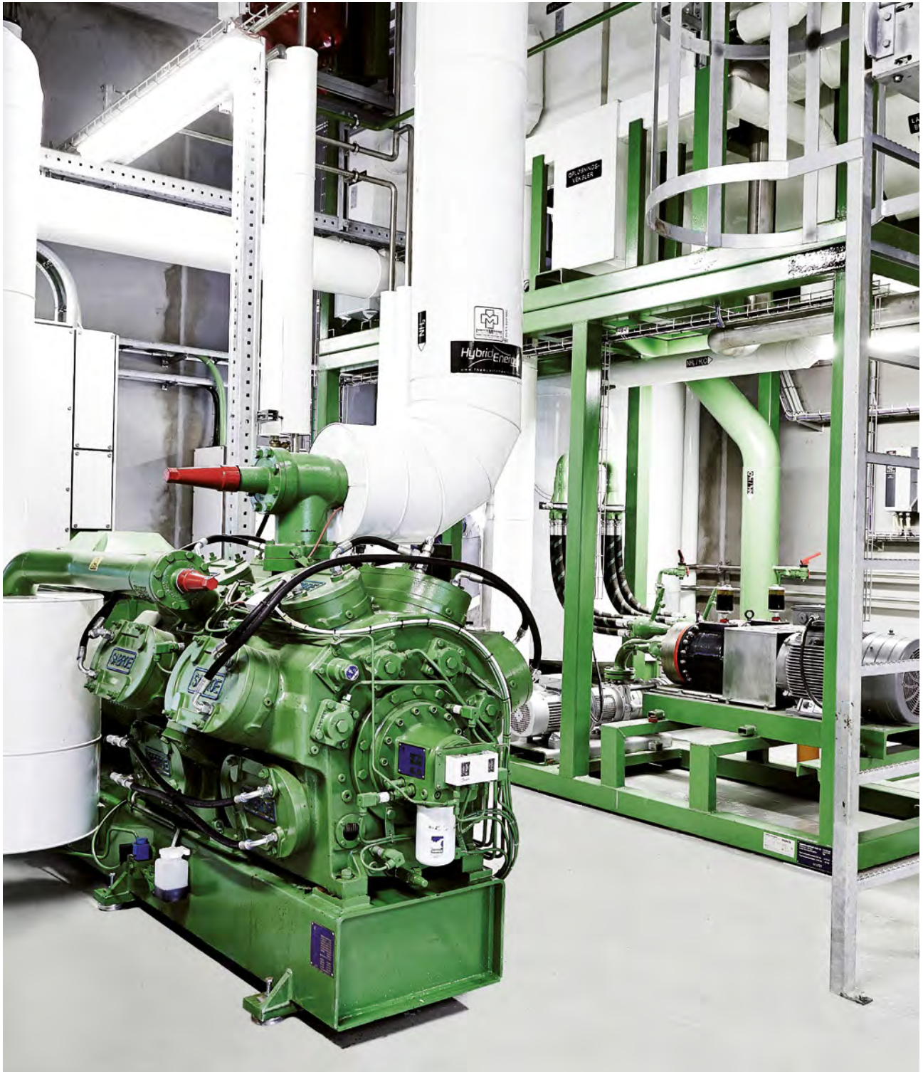
Figure 6: Heat pump installation at Arla Videbæk dairy
