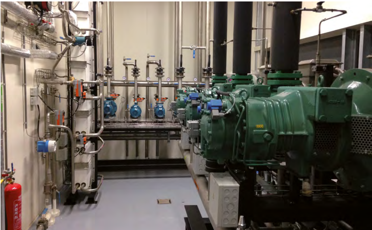
Figure 5: Heat pump installation at Hutten slaughterhouse
