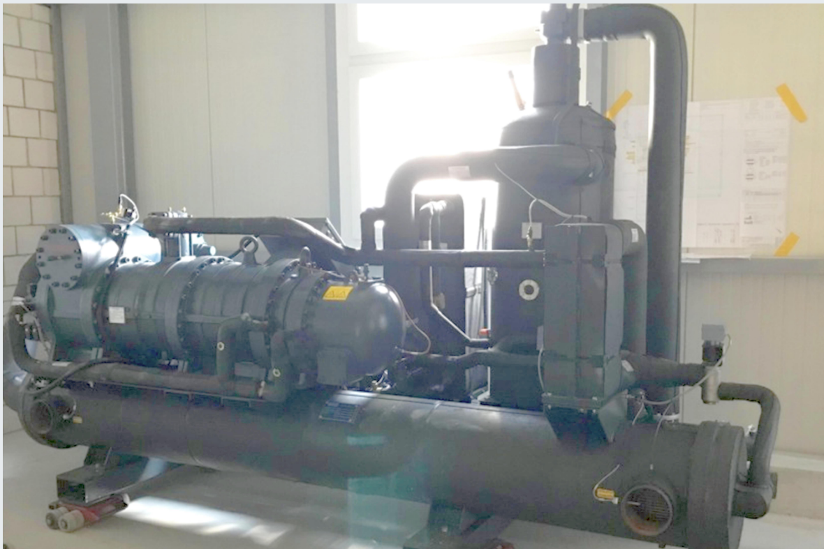
Fig. 2: High temperature heat pump installed at the technical room of the mountain cheese factory [4]. The mildly flammable refrigerant R1234ze(E) demands special measures for fire protection and escape routes.
