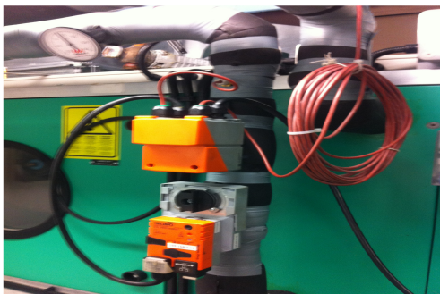
The Belimo Energy Valve controls the supply of cooling water for the air conditioning heat exchanger.
